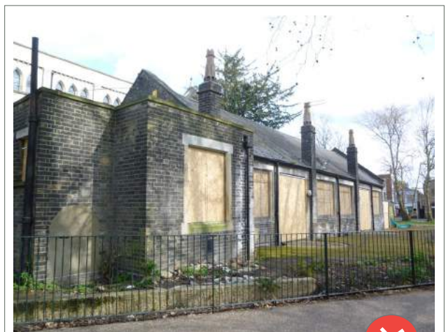
Examples of buildings in Bruce Grove and Tottenham Green Conservation Areas that have fallen in to disuse can be in danger of neglect.
